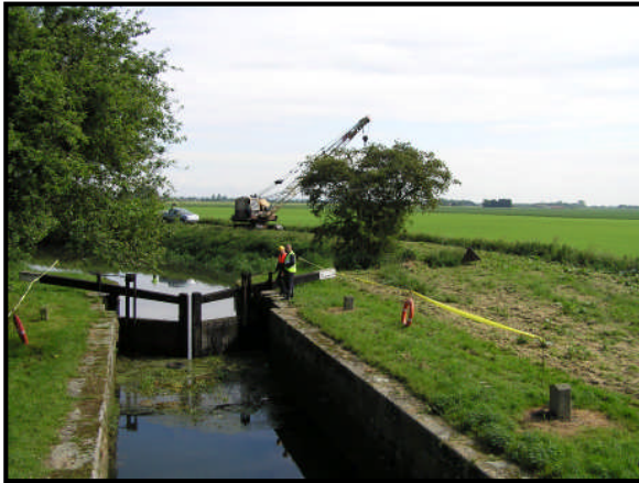
The arrival of the crane. One hour delay due to fault on compressed air controls.
